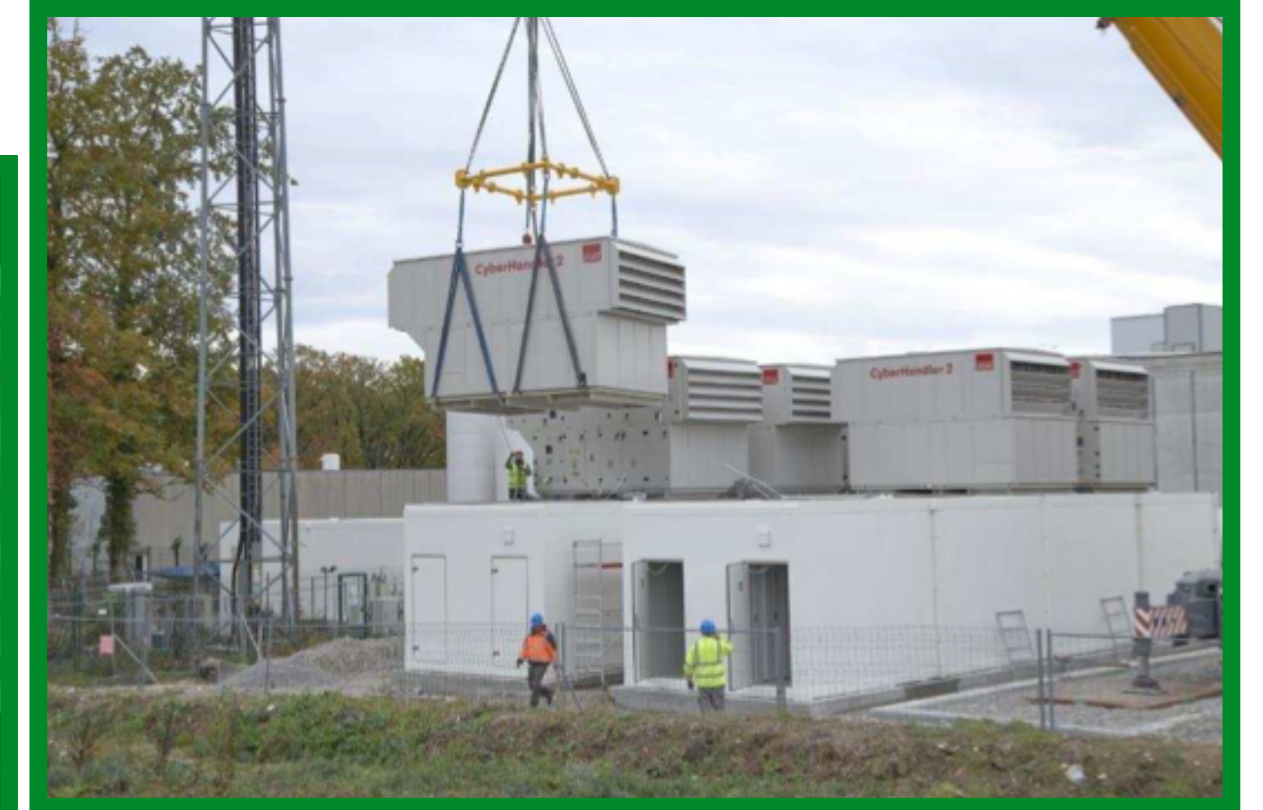
New data centre
